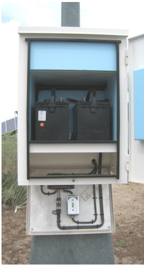
Interior showing Insulated Tank, Battery Compartment and Electronic Compartment with Drop-down Panel.
